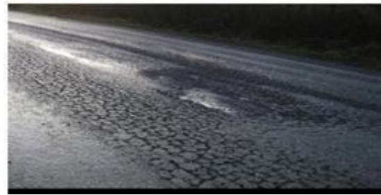
Fig.1.2. Mixed ratio damages
