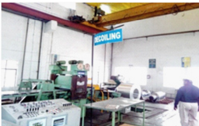
Photo 1: Decoiling & levelling processing section
