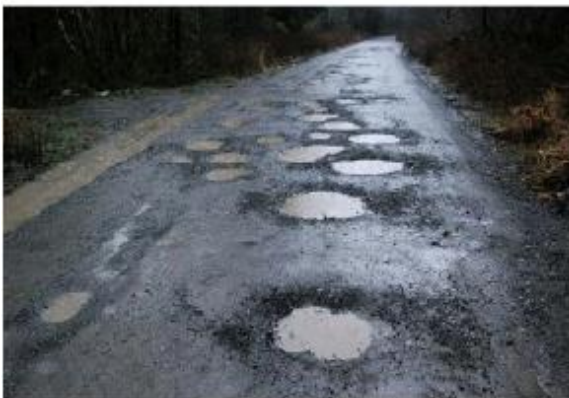
Fig.1. Condition of road with potholes
